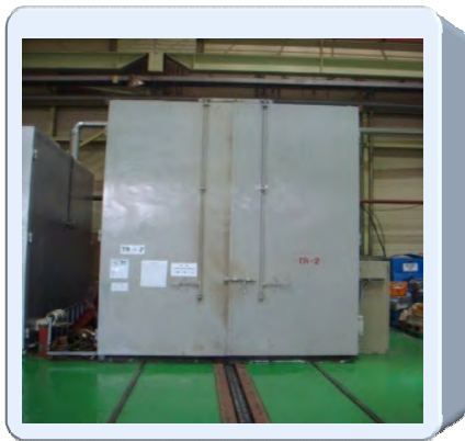
LARGE DRYING FURNACE
